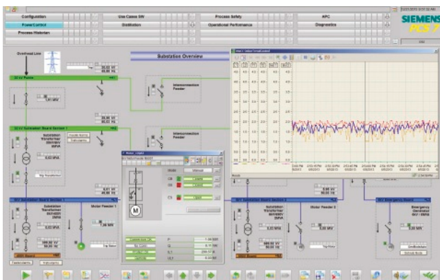
Example of a plant display for medium-voltage switchgear with trend window and faceplate of a medium-voltage motor
